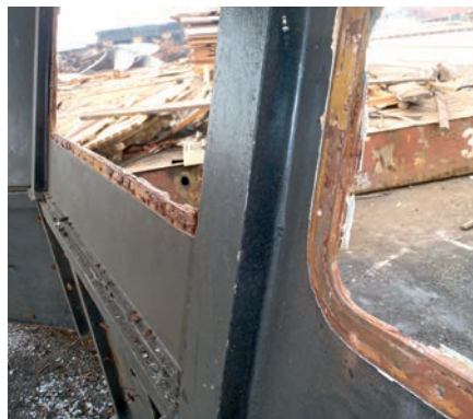
PCB-containing material had to be recovered carefully from the window frames of the wheelhouse as the 'SS Bekalang' was recycled.
