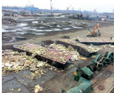
Sea2Cradle managed the breaking of the 'SS Bekalang' last year at the Changjiang yard in China. Here, insulation is removed from tank walls.
