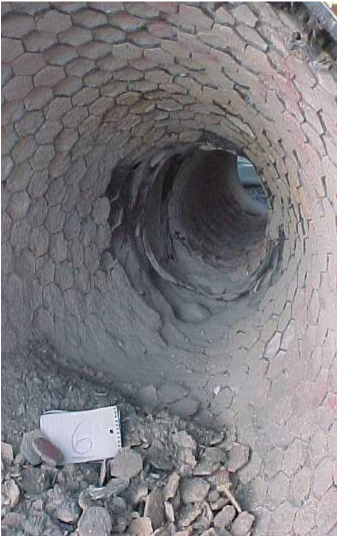
Dustbowl refractory loss
