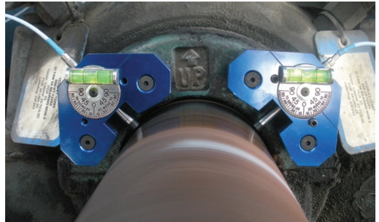
Figure 4: ID fan with the removable proximity probe mounts installed on the bearing housing
