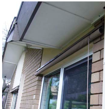
↑ External blinds on the east-facing windows keep the sun off the glass on hot summer mornings.
