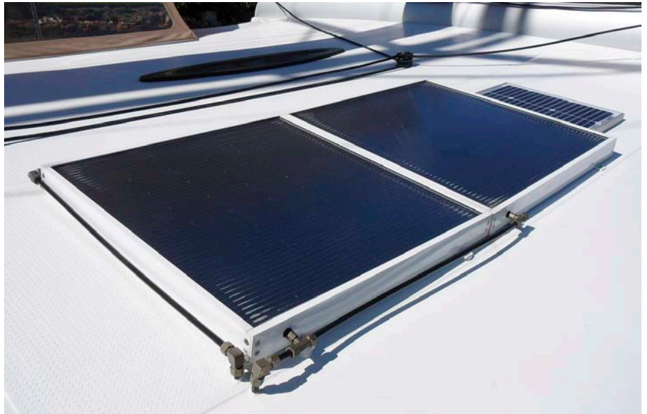
↑ Hot water is provided by two Heliatos solar collectors and circulated by a pump run by the 10-watt solar panel.
