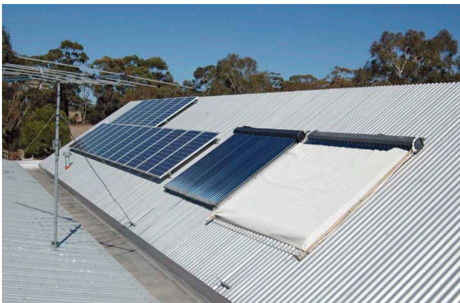
↑ Around 3kW of photovoltaics sits next to the solar water heater, which supplies hot water for domestic use as well as the in-slab hydronic heating system. It's backed up by an efficient wood-fired boiler. During summer, one of the water heating collectors is covered to prevent overheating, as seen here.
