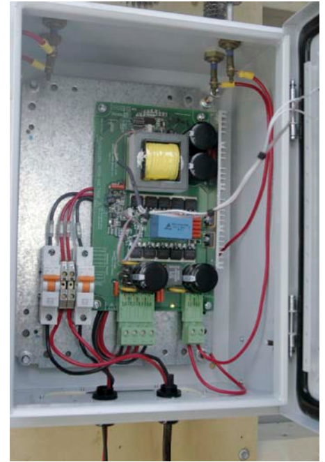
↑ The turbine produces power at 75 volts which is stepped down to 27 volts for the batteries.
