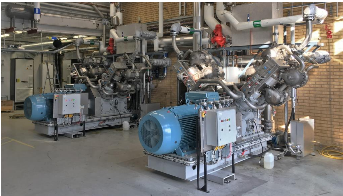
Figure 3. Two of the three heat pumps currently installed at AstraZeneca’s R&D facility in Gothenburg, Sweden. Heat is transferred to the heat pump from the heat recovery circuit and steam is delivered from the heat pumps’ steam generators to the steam distribution system. The third heat pump is installed on the opposite side of the room.
