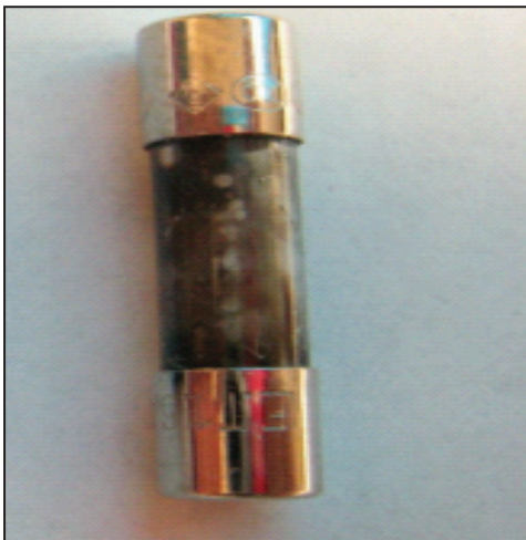
< Fuse, F901 > Can look at physical condition.
