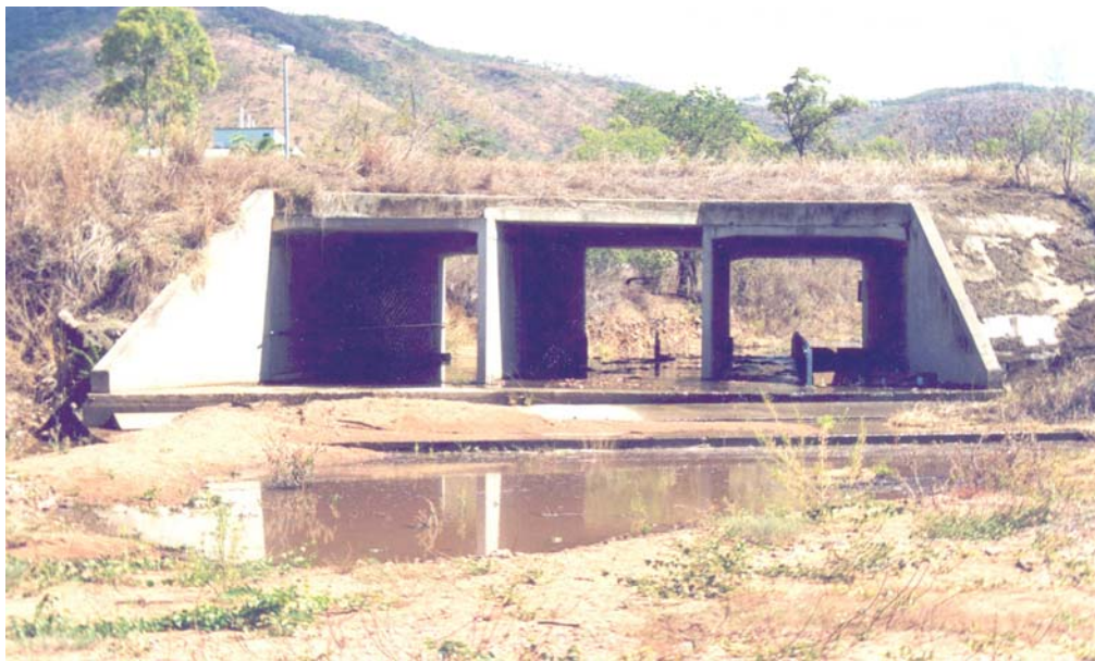
Figure 2.6 Campus Creek at the start of Wet Season rains, December 2002 (Note: fishway in R.H. barrel of culvert)
