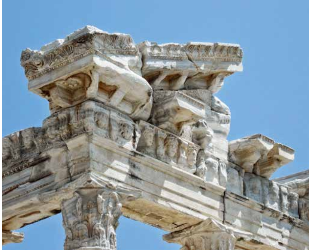
FIG. 5. The entablature of the Temple of Apollo at Side, northwest corner, after A.D. 114
