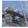
Partial reconstruction (work in progress) of the Parthenon, Athens, to ensure structural stability, 2007
