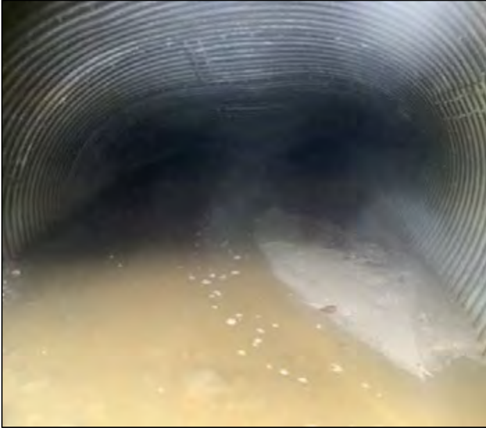
Photo 1. Facing outlet, culvert collapsed in centre
