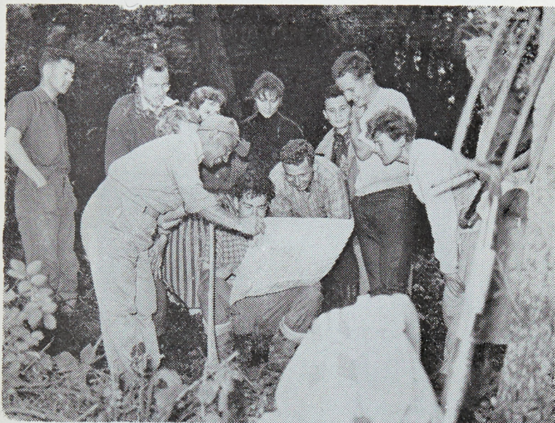
Members of I.V.S. check draining maps on the site of the new Cheshire Home at Ferguson Common, Penn, Wolverhampton, where they have been preparing the site for the building.
