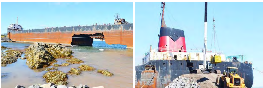
The wreck and the demolition site © Laura Jean Grant - Cape Breton Post
