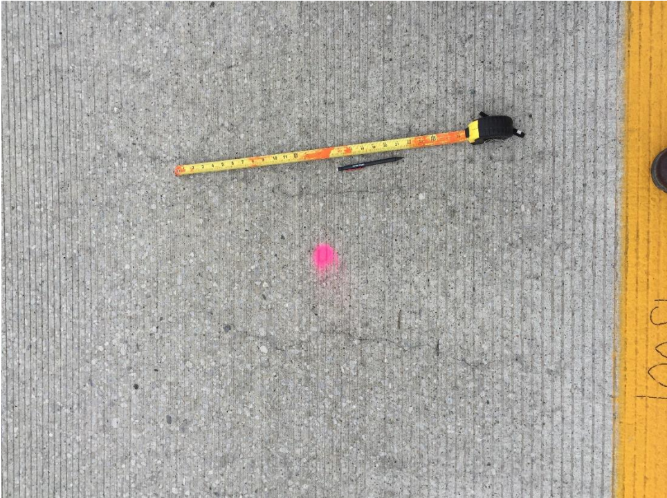
Figure 42. Cracking on southbound, inner lane of the normal concrete deck
