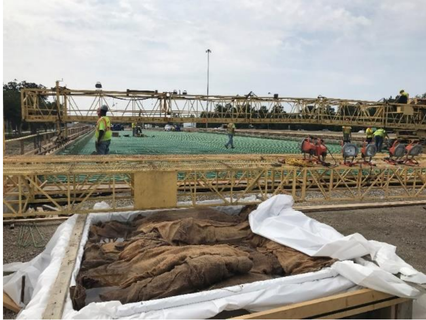
Figure 27. Bridge prior to deck placement, with wet burlap ready to be placed
