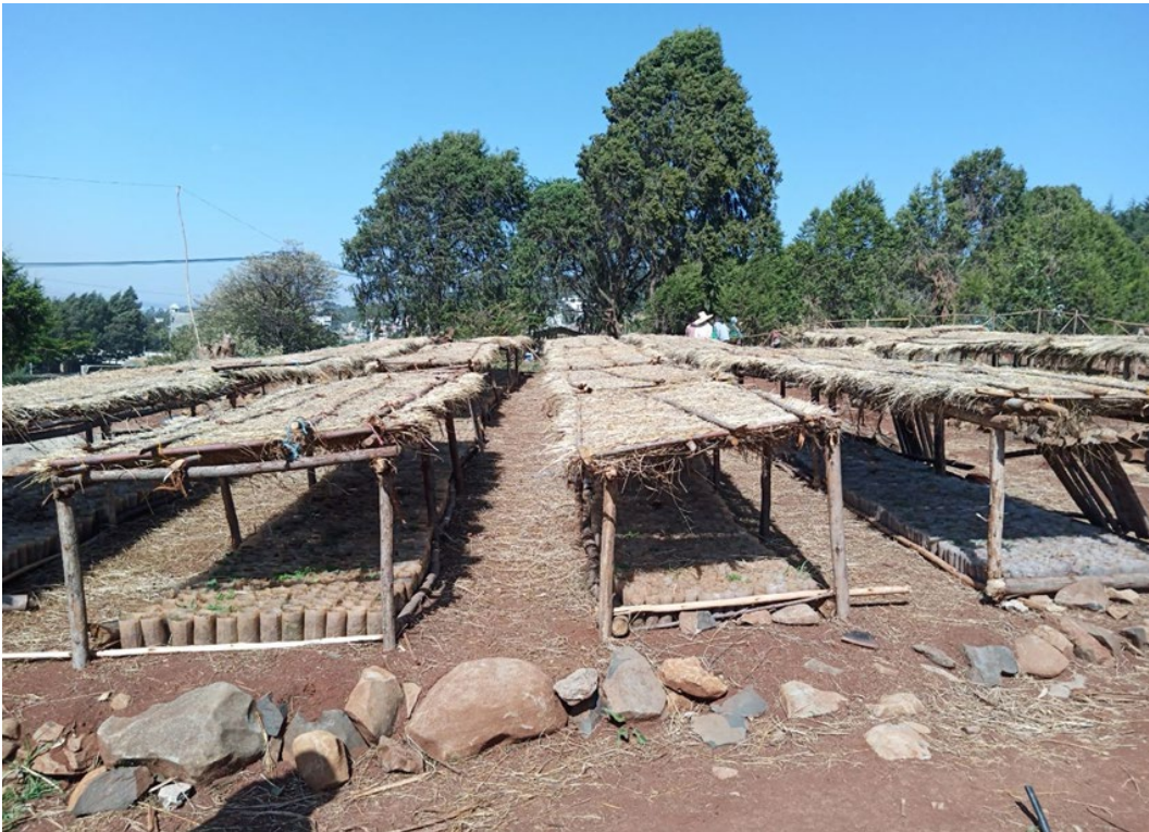
Fig. 6. Shades constructed to protect seedlings from sunlight after propagation (this shade has been constructed in the garden not only for this project but also for future use in coordination with other stakeholders).
