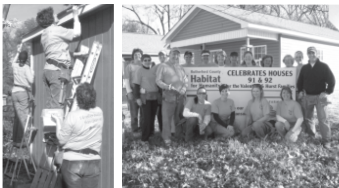
Rutherford County associates help build a home during Habitat for Humanity's Women's Build weekend.
