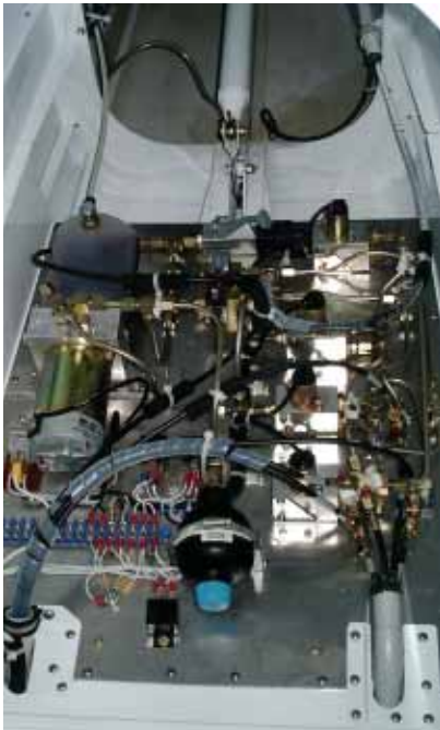
The electric and hydraulic components of Roth's retraction system are plate-mounted in the plane's baggage area behind the rear seat. If necessary, Roth can conveniently pull the whole system out as a complete unit.
