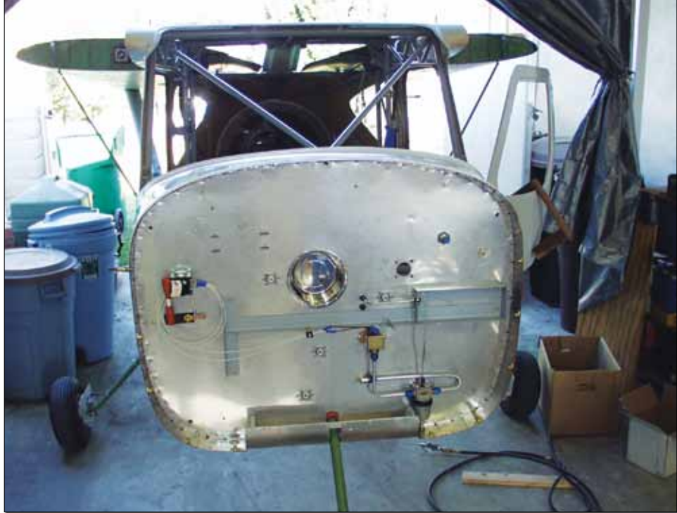
This GlaStar firewall shows eyeball fittings for cables, added support for an oil cooler and a "dog bowl" indentation to allow clearance for a prop governor.
