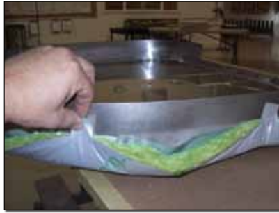
Non-flammable sound-blanket material is attached to the cabin side of the firewall before it is pushed into place at the Glasair Customer Assembly Center.
