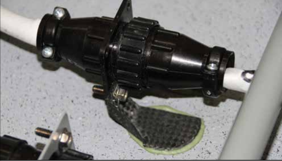
A spoon standoff used to mount cable connectors to the floor of the cabin.
