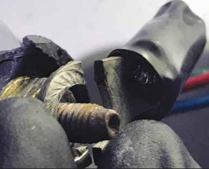
Overtightening an oversized lug does not prevent failure. This one eventually broke off at the alternator. You can see the distortion marks on the lug from overtightening it.
