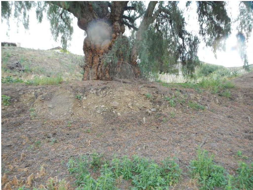
FIGURE A-6. TREE GROWING AT EMERGENCY SPILLWAY ENTRANCE
