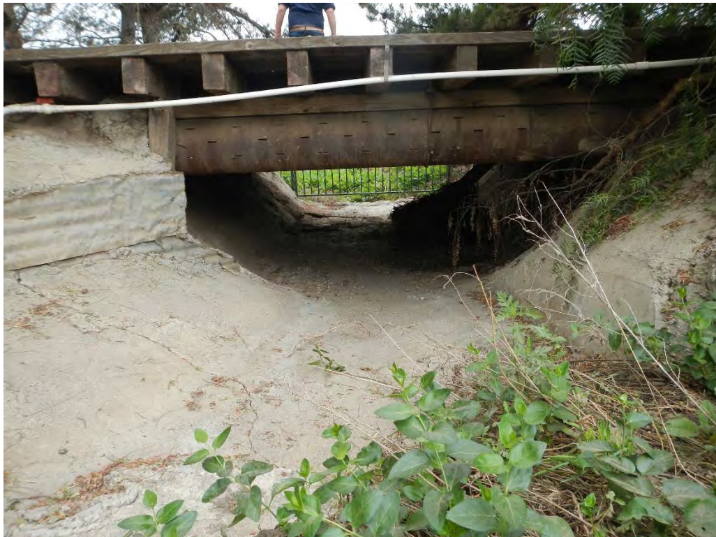
FIGURE A-16. UN-NAMED FARM ROAD CULVERT CROSSING AT 90-DEGREE BEND
