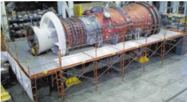
Gas turbine for Combined Cycle Power Plant
