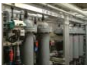
Kichijoji store: Groundwater membrane filtering system
