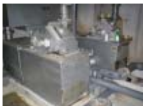
Fuchu store: Underground pump for waste water
