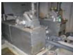
Fuchu store: Underground pump for waste water
