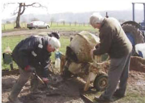
North Wales club members doing the jobs that keep them in the air, laying the base for a new LPG tank
