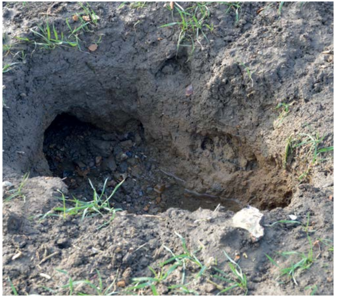
The collapsed drain led to this hole appearing in the soil surface.
