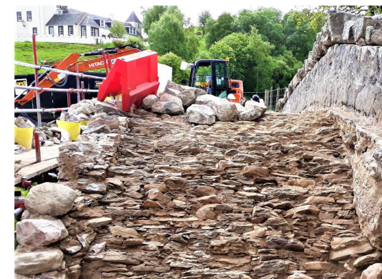
Fig. 9 Tordarroch Bridge repair in 2022 after a parapet collapse – Note the traditional, undressed, arch ring top of tightly packed thin stones under the roadway after c.240 years in service ©The Highland Council
