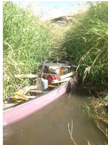
Post pounder access and transport can present a unique challenge. Left: hydraulic post-pounder is transported using a canoe. Pataha Creek, WA.
