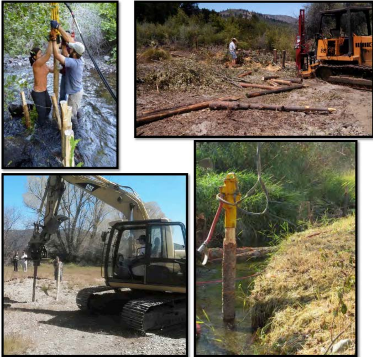
Figure 27: Hydraulic post pounder options. Options include, clockwise, starting from upper left: (a) a hand-held pounder attached to hydraulic power pack, (b) a post pounder attached to bulldozers, (c) a handheld pneumatic post pounder attached to an excavator and (d) a modified excavator with a vibrating pad. Options (a) and (b) take approximately 5 to 10 minutes per post, depending on substrate, and it can be difficult to get to the desired depth. Option (d) takes less than 1 minute per post and can drive posts as deep as needed. All pounders have a metal cylindrical cap that holds the post in place while pounding. Each option has pros and cons to consider, including cost, maximum depth the posts can be pounded, substrate type, operator strength and expertise, and the amount of likely riparian and instream disturbance. Photo credits: (a) Nick Weber, Ecological Research, (b) Mark Cookson, USFWS, (c) Peter Thamer, Siskiyou County Resource Conservation District, and (d) Julie Ashmore, Okanogan Highlands Alliance.
