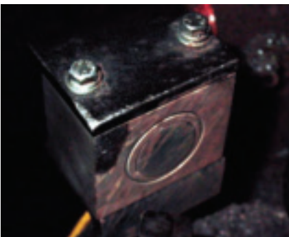
Fig. 4 — This prox sensor installed in a bunker block is well protected from heat, slag, and impact.
