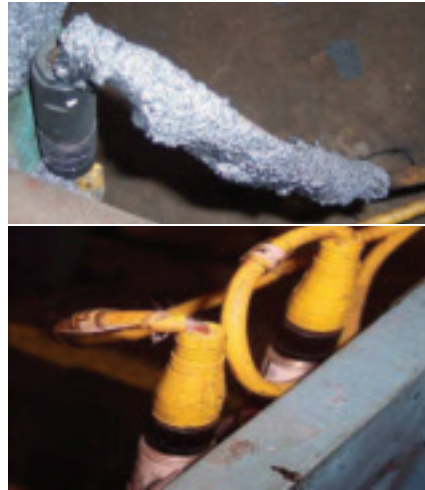
Fig. 5 — These unprotected connections were destroyed by slag, heat, and impact.
