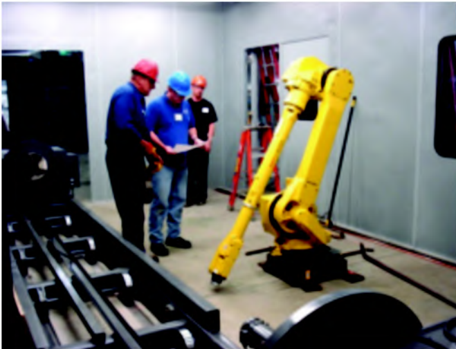
Staff and contractors from Stork Cellramic prepare the high velocity oxygen fuel spray chamber and robotic arm for installation.
