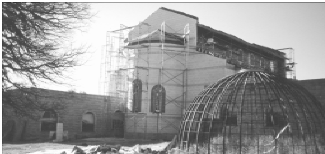
Holy Archangels Greek Orthodox Monastery in Kendalia, Texas, formerly a Muslim retreat, is in the process of completing the dome of its new church.
