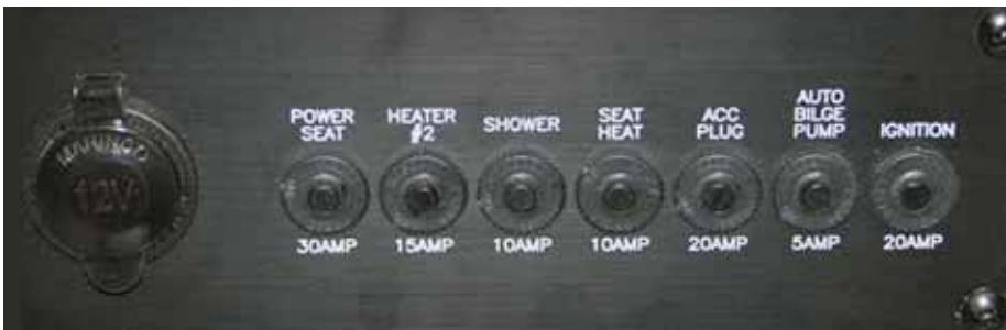
Figure 2-13. Circuit Breaker Panels
