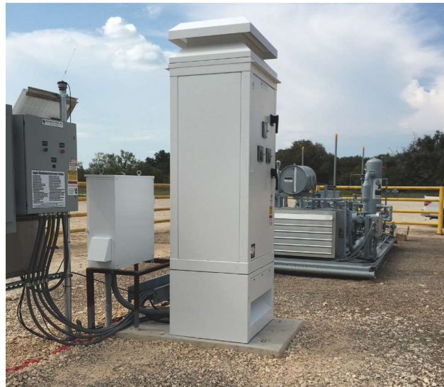
The electric-driven wellhead gas-lift compressor in the background is powered by VFDs located in the tall white cabinet. Compressor operations are controlled by a PLC in the far left gray cabinet. (Source: Encline)
