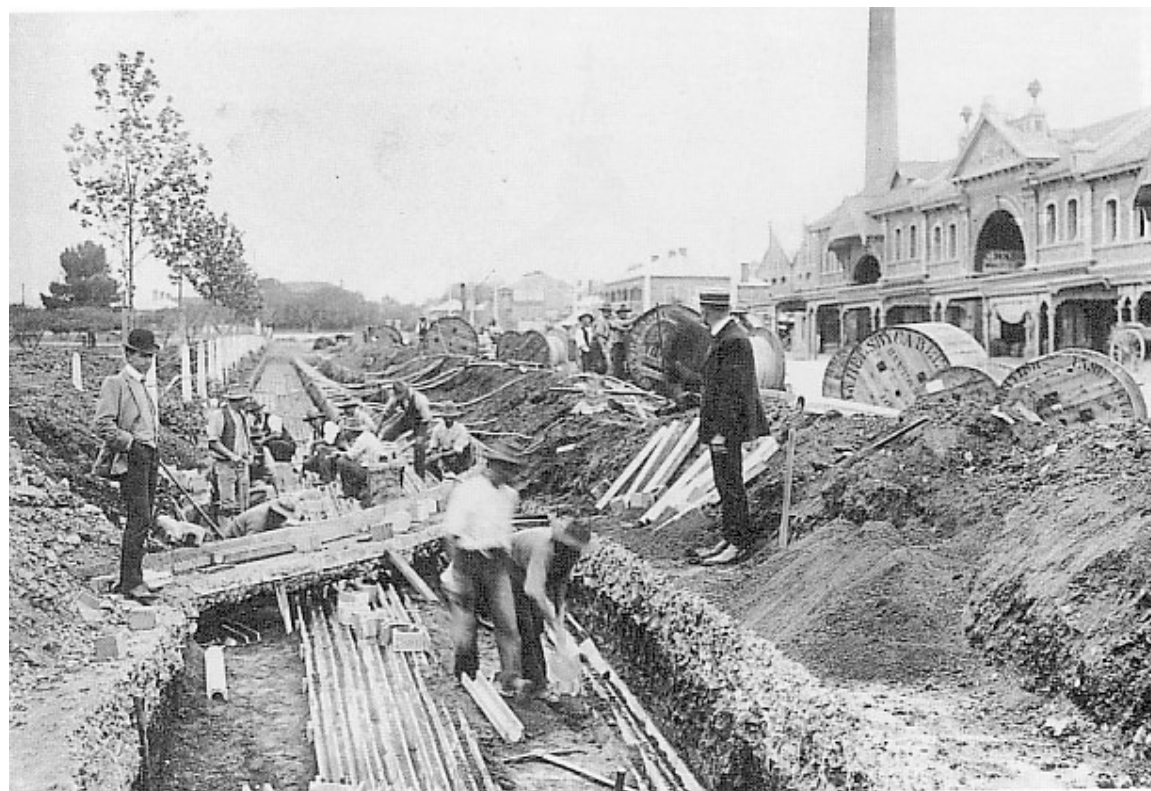
Figure: Laying electricity cables in East Terrace in 1907-08. Note the white painted post and wire fencing and the young Plane Trees ( Platanus orientalis ) to the left. Source: ACC Archives.
