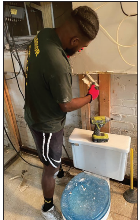
Julius Wilkerson helping repair a bathroom in a home that had flood damage.
