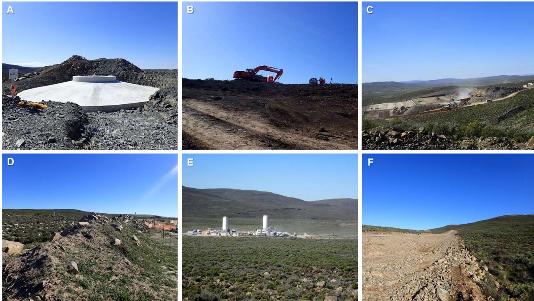
Figure 5-2 Photographs illustrating potential impacts associated with the construction of Wind Energy Facilities. A) Installation of turbine base into ground achieved through blasting and use of heavy machinery, B) Earthworks using heavy machinery leading to noise and vibration pollution, C) Construction of substation involving clearing of vegetation and reshaping of topography through use of heavy machinery, D) Poor topsoil stockpiling practices leading to reduction in topsoil quality, E) Cement plant and poor stockpiling of source material leading to dust pollution into adjacent natural areas and F) Clearing of vegetation for road network.
