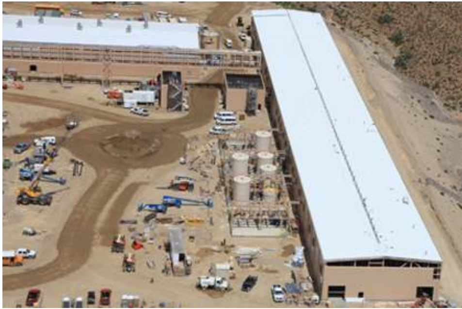
Figure 5 Picture of a typical Rare Earth Separation Plant
