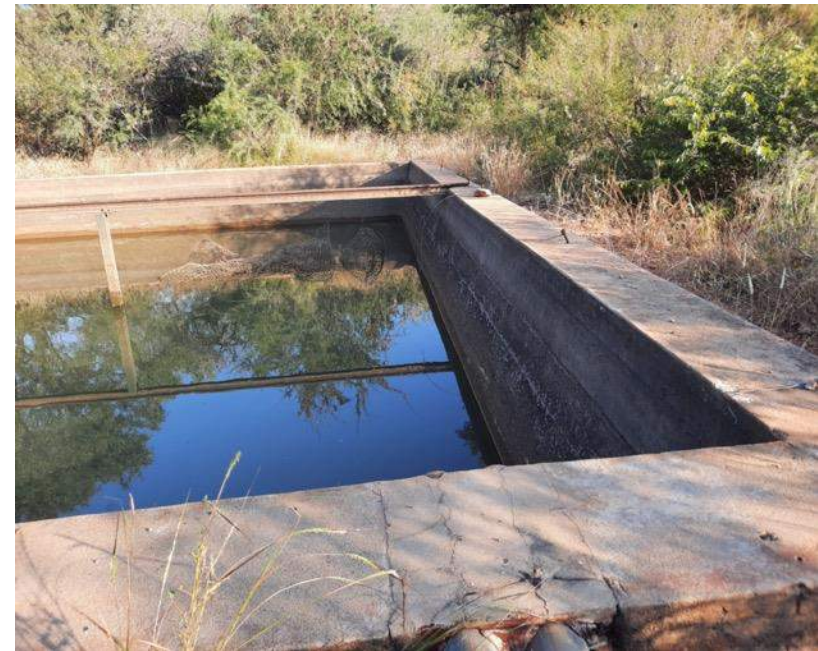
Figure 36 – Large cement water reservoir at Site 2-5
