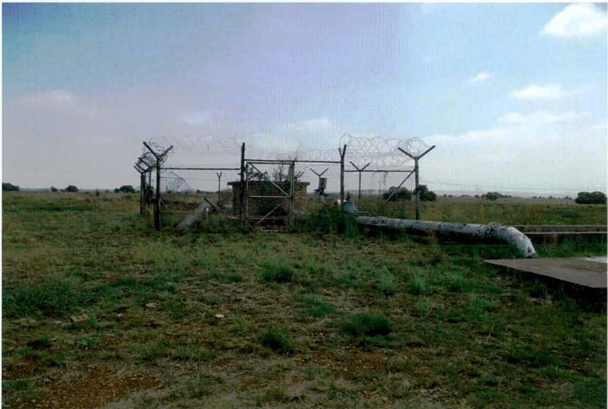
Figure 8: Mine water booster pump next to point B.
