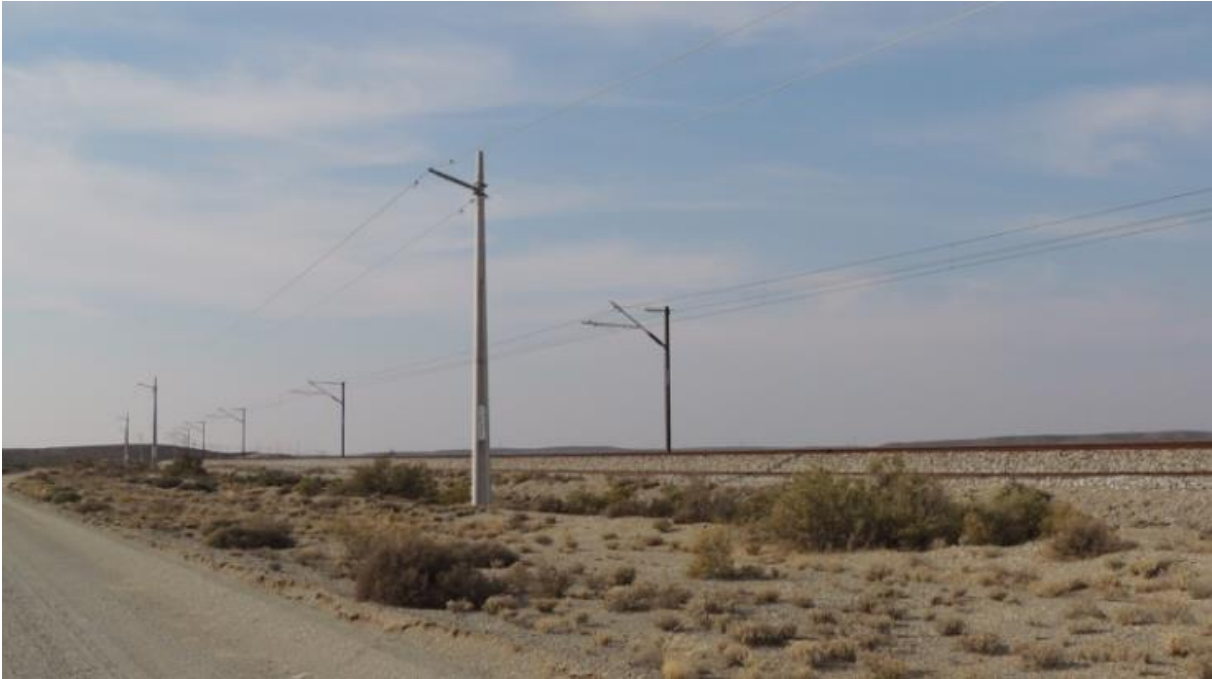
Figure 14: Photograph of the overhead electrical structures and cabling associated with the Shishen – Saldanha railway line.
