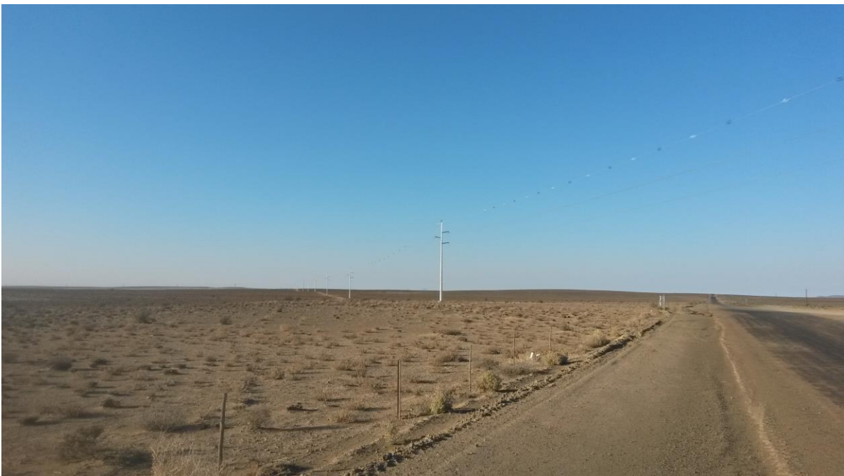
Figure 4: A photograph of a typical single-circuit monopole type structure. Bird diverters (alternating black and white) can be seen on the line
