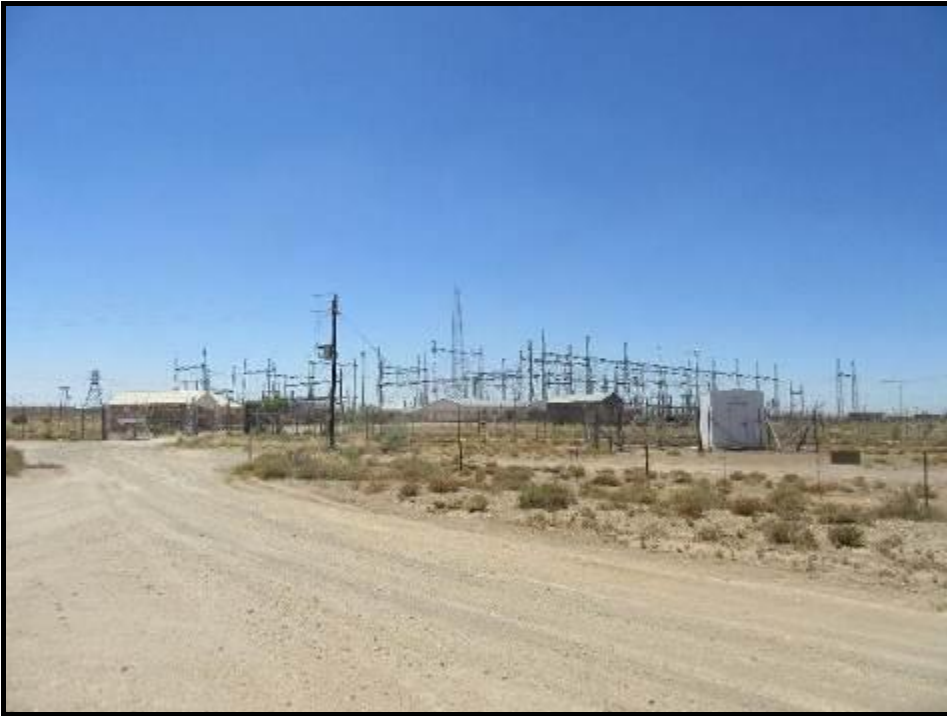
Photograph 1.3 Eskom's Helios substation adjacent to the Nuwepos Road
