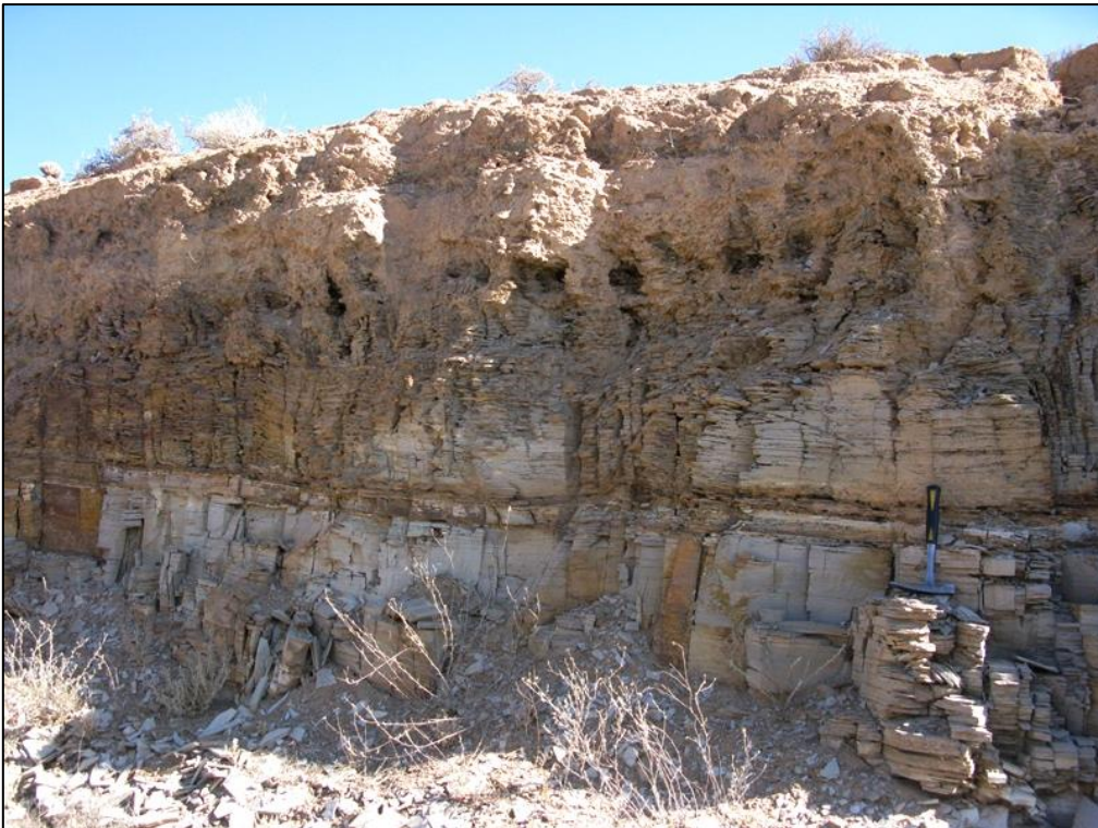
Figure 13: Borrow pit cut face section through gently-dipping, tabular-bedded mudrocks of the Whitehill Formation overlain by saprolite and thick, silty, gypsiferous soils (Loc. 261) (Hammer = 30 cm).
