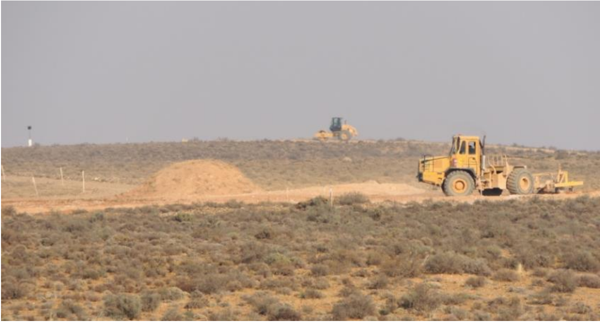
Figure 17: Earth moving vehicles currently on site for the construction of the Mainstream WEF.
