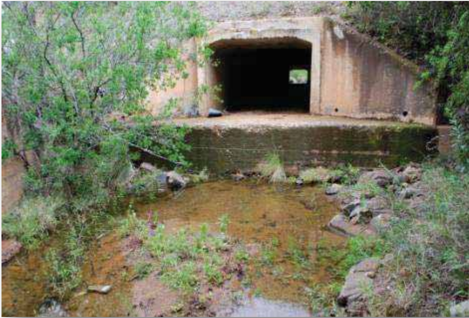
Plate 2: An example of an elevated culvert that as raised the level of riverbed resulting in a form of habitat fragmentation
