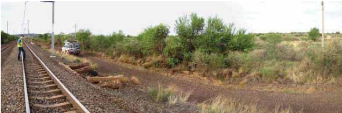
Figure 30: Illustrates a culvert crossing in the central section of the Glosam loop; a man-made channel has been made to drain sheetwash away through the raised embankment and culvert, the channel disappears downstream of the railway line crossing.
