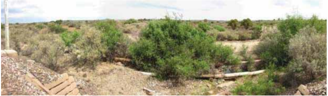
Figure 20: Illustrates a culvert in a wash crossing (map label 24) west of the Tsantsabane area. No distinct channel features or scour marks are evident up and downstream of the culvert, but a linear drainage system is distinct on available aerial imagery.
