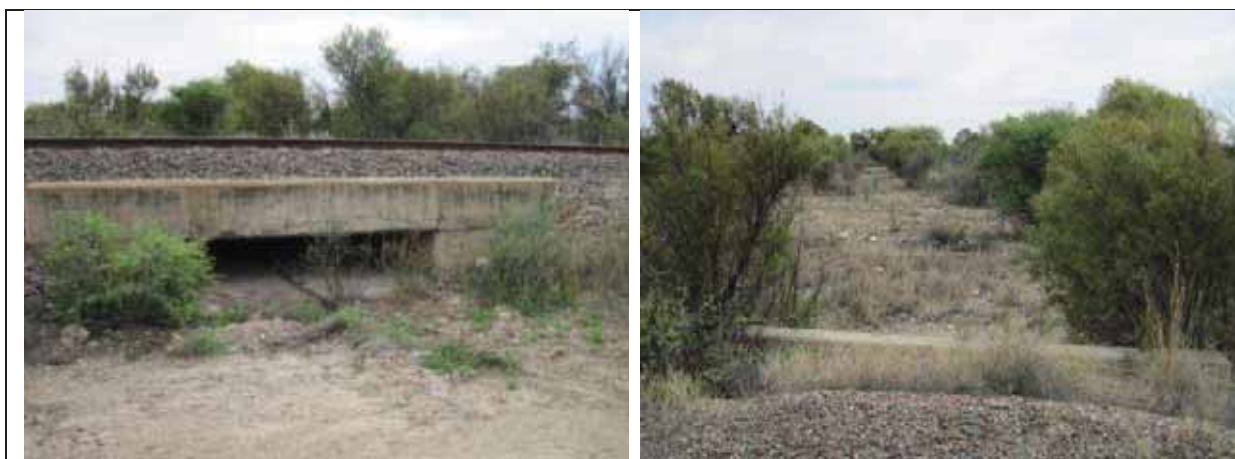
Figure 14: Illustrates a culvert and portion of a wash located adjacent to the Ulco area (map label 12); the wash is not well defined, but is located in close proximity to the loop extension. No channel features or signs of scour erosion are present upstream or downstream of the culvert.
