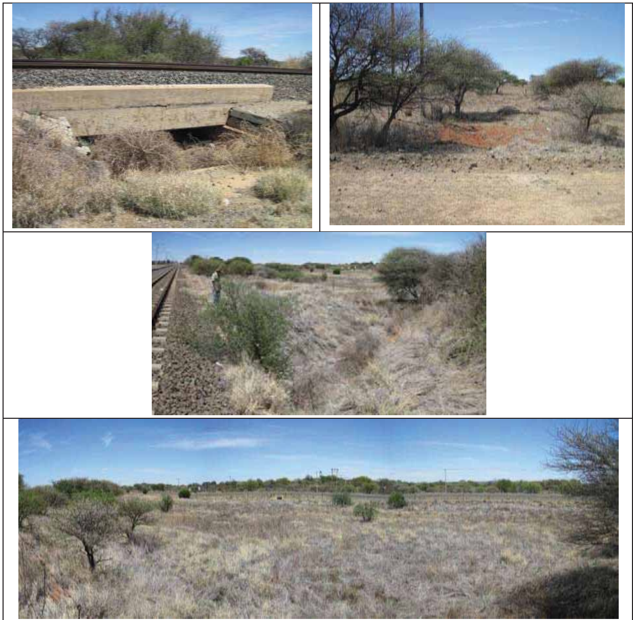
Figure 4: Illustrates the Beaconsfield drainage line 1 crossing with its existing culvert (top left), indistinct channel development upstream of the loop (top right), created channel on the raised embankment downstream of the loop (center), and indistinct channel further downstream towards the road crossing (bottom).
