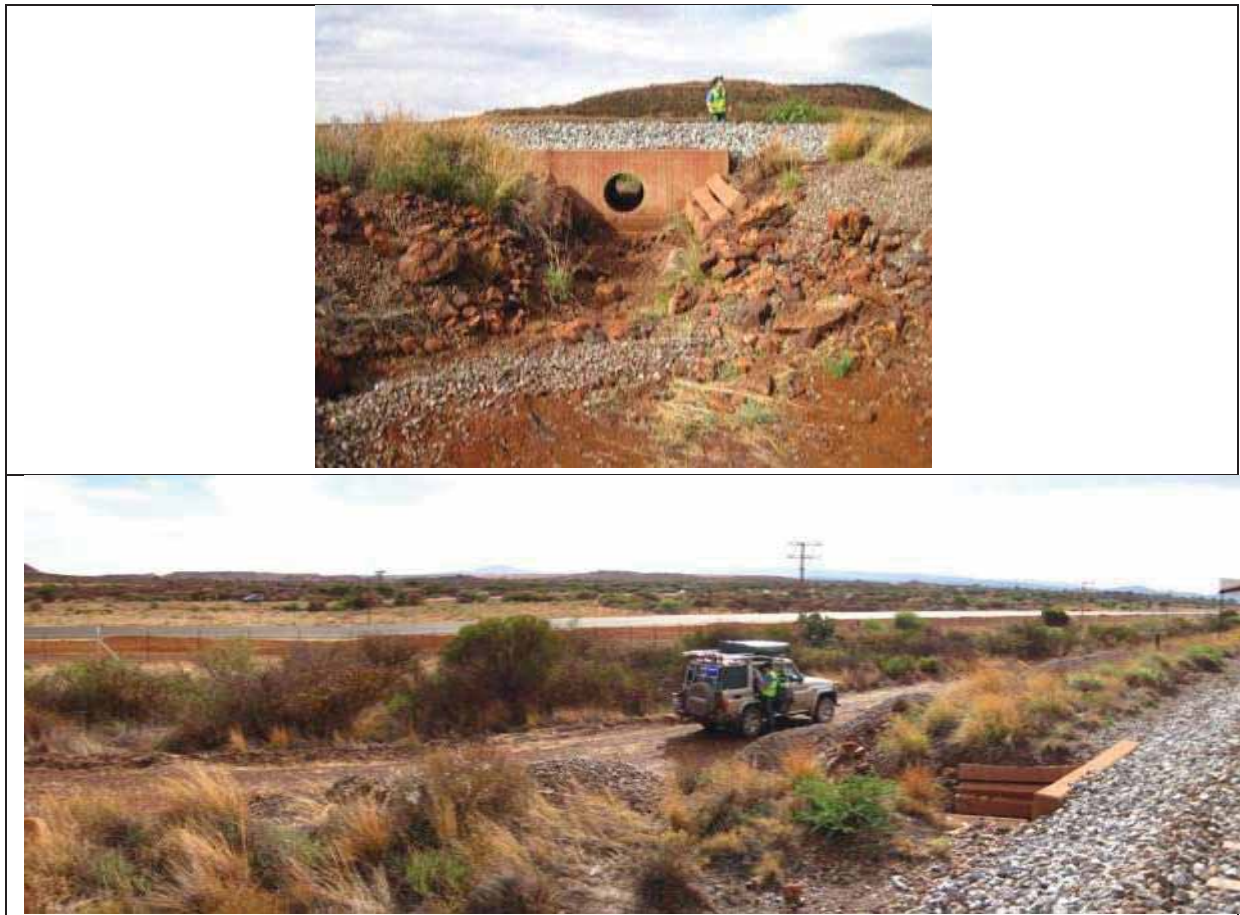
Figure 27: Illustrates a pipe crossing in the far western section of the Postmasburg loop (top and bottom). No natural watercourse or drainage line feature, including a natural channel, occurs at this point (bottom); the perched pipe and human intervention has resulted in man-made channel-like feature in the embankment of the railway line (top and bottom).
