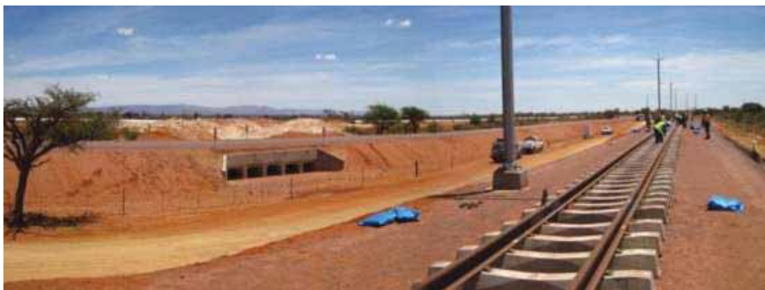
Figure 34: A set of culverts and newly created downstream channel in the center of the Sishen loop section, with no watercourse or drainage system present.
