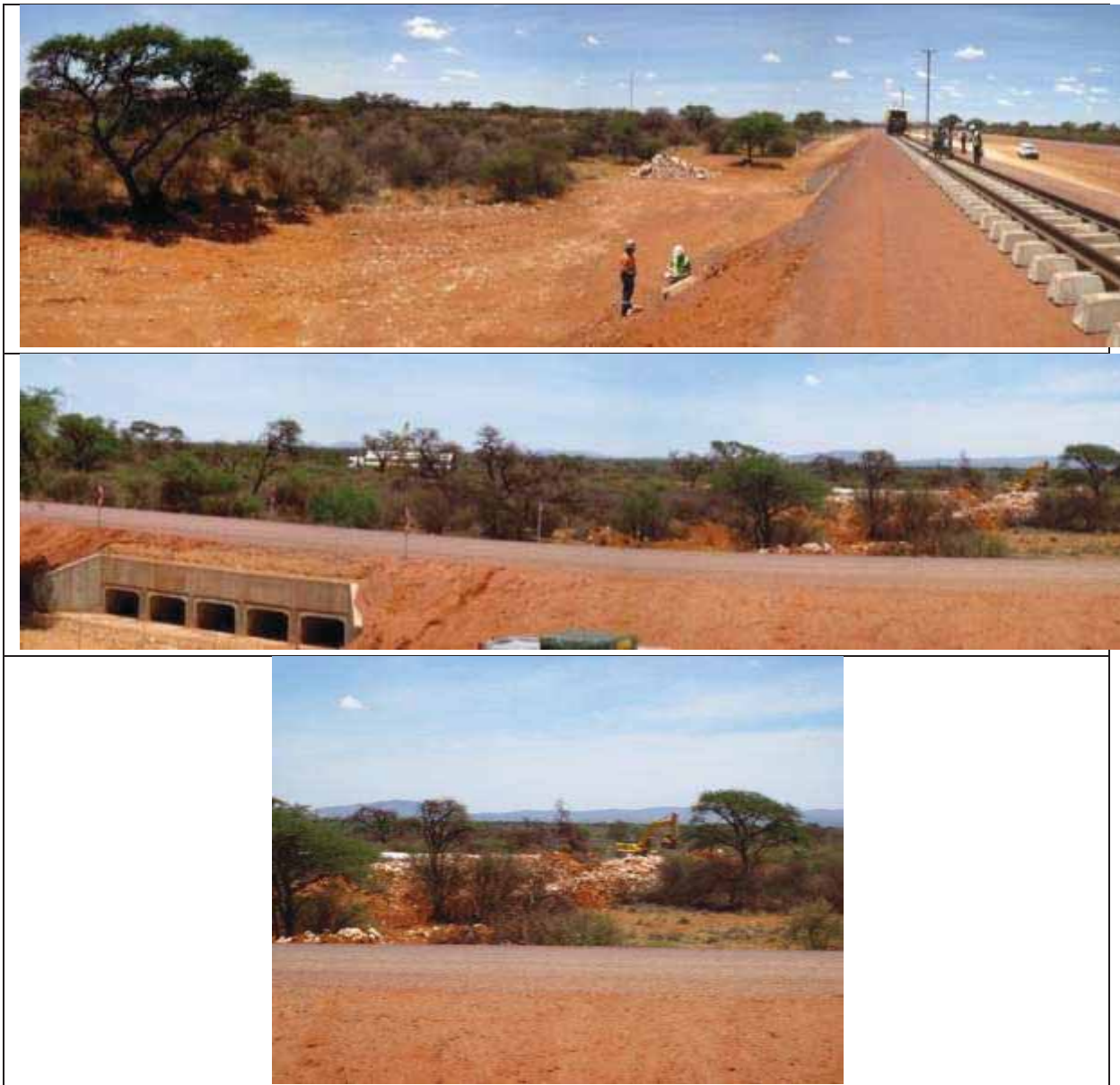
Figure 33: Illustrates the upstream (top) and downstream (center and bottom) sections of a flat drainage system crossing in the south-eastern section of the Sishen loop. The system has been recently impacted by a new railway line and road crossing associated with the Sishen West Expansion Project (top and centre), while a channel has been excavated downstream thereof (bottom).
