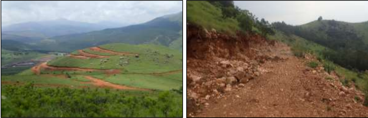
Figure 6: Recent activities that directly impacted on floral habitat within the focus area mainly included the construction of prospecting roads as part of exploration activities and dumping of soil discard and rock material.
