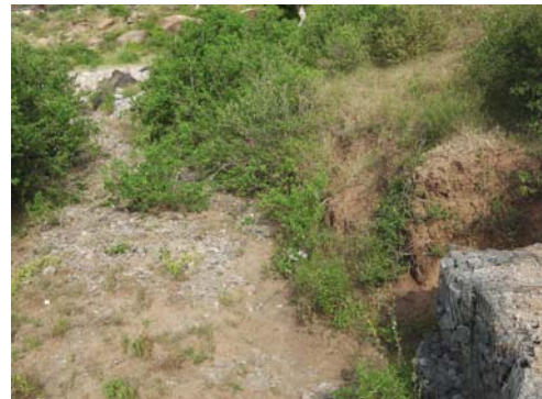
Figure 71: Erosion associated with the roads and culverts.
