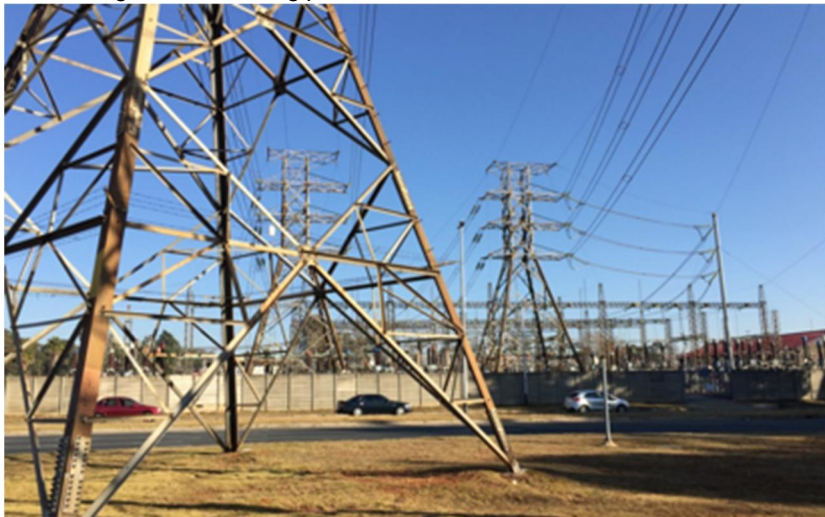
Site Photo 7: View west of the point where the proposed power line enters into the existing Hamberg Road Substation adjacent to existing power line.
