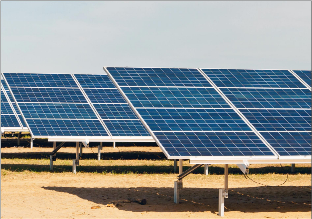
Figure 5: Photographic example of typical fixed PV arrays (Jasper Power Company, 2014).
