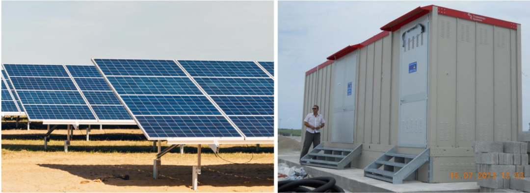
Figure 6: A typical example of installed Solar Photovoltaic Panels and Container Substations which will be used at the SR PVP project
