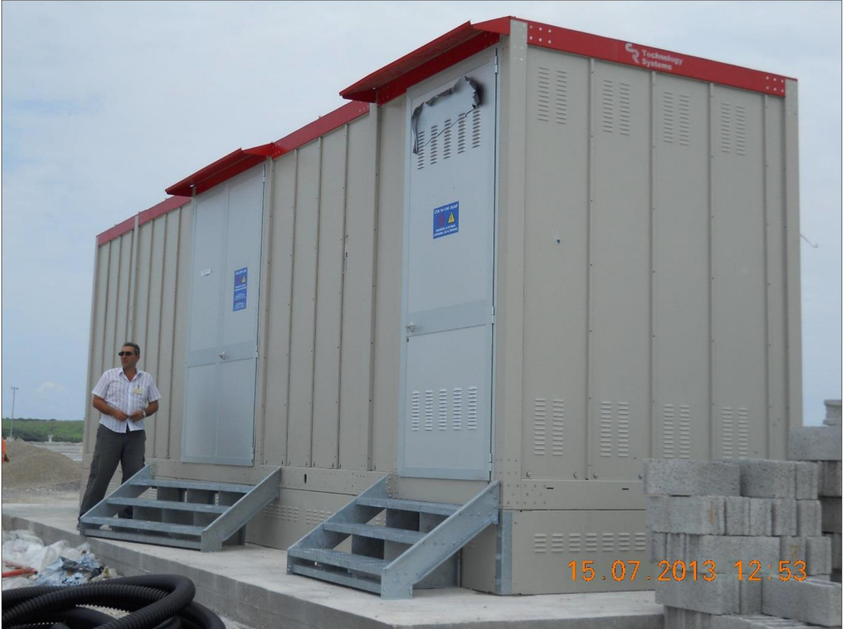
Figure 6: Photograph of a typical containerized substation (Source: SolarReserve, 2013)
