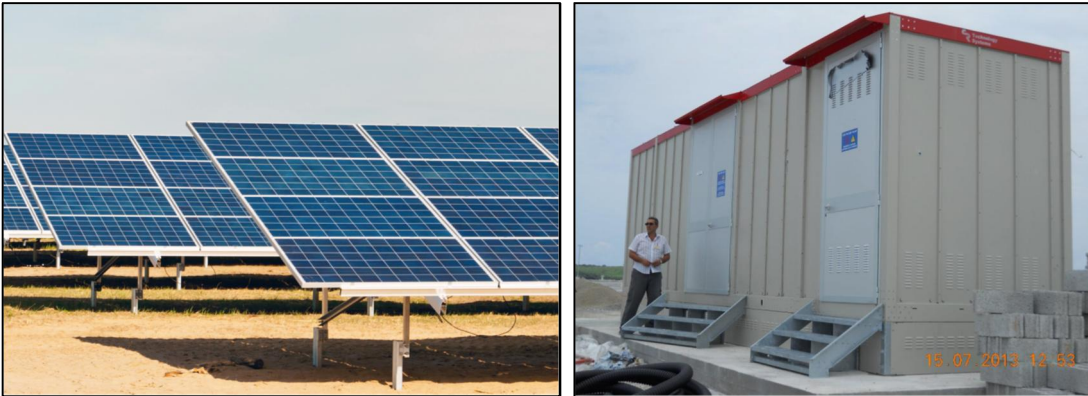
Figure 8: A typical example of installed Solar Photovoltaic Panels and Container Substations which will be used at the SR PVP project
