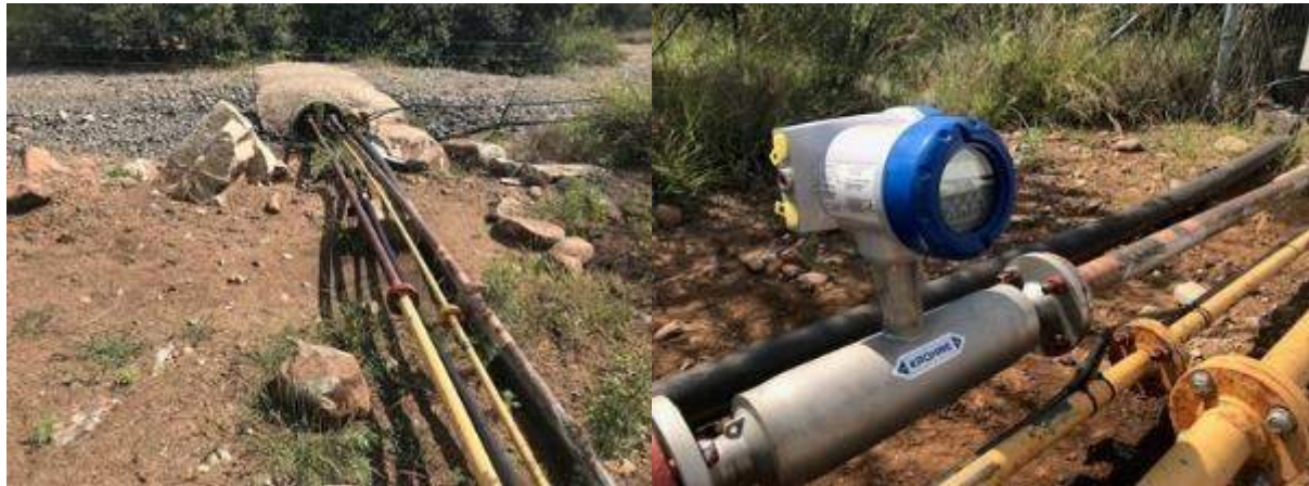
Photo 6: Supply pipes and flow meters
