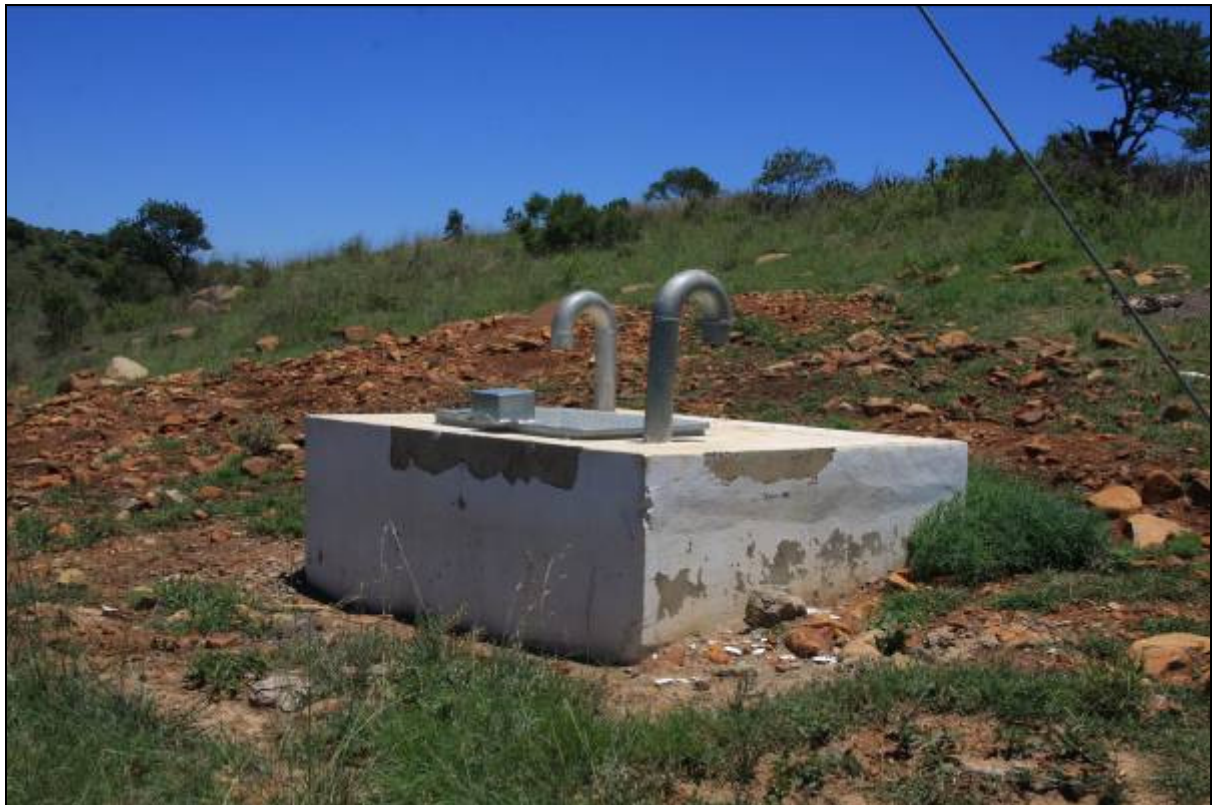
Plate 6. Air valve chamber on an existing pipe line. These will be required at certain positions along the entire length of pipe line.
