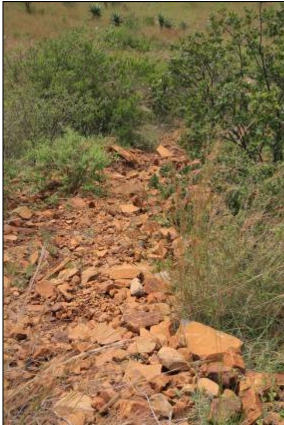
Plate 25. Excavations for a pipe line that has not undergone rehabilitation and is exposed to significant erosion.
