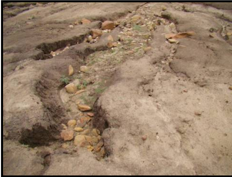
Figure15. Extensive surface, rill and gully erosion occurs adjacent to the proposed road alignments.
