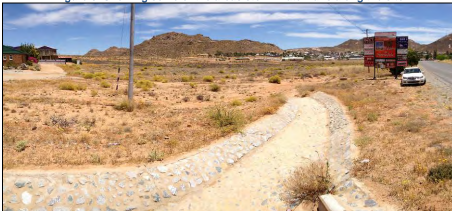
Figure 7: Already formalized storm water drainage from adjacent properties running onto the site.
