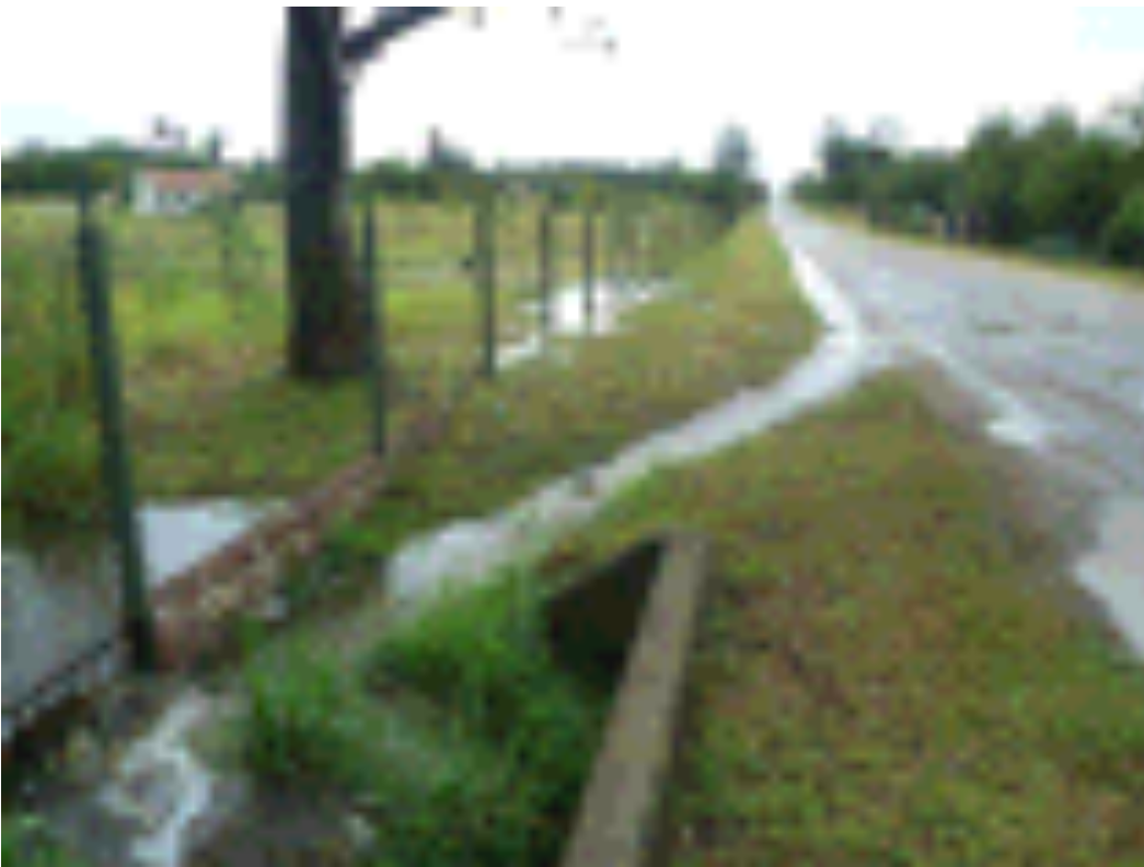
Figure 22 Culvert under Mc Innes road receiving water from the road itself (1 hour after a storm event on the 31 st of January 2014)
