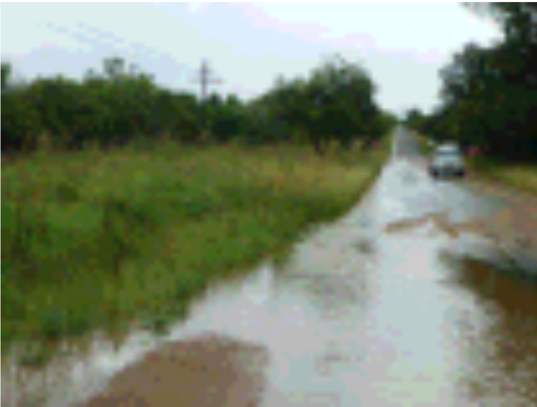
Figure 29 Storm water still present in Zinnia Road one hour after a storm event on the 31 st of January 2014
