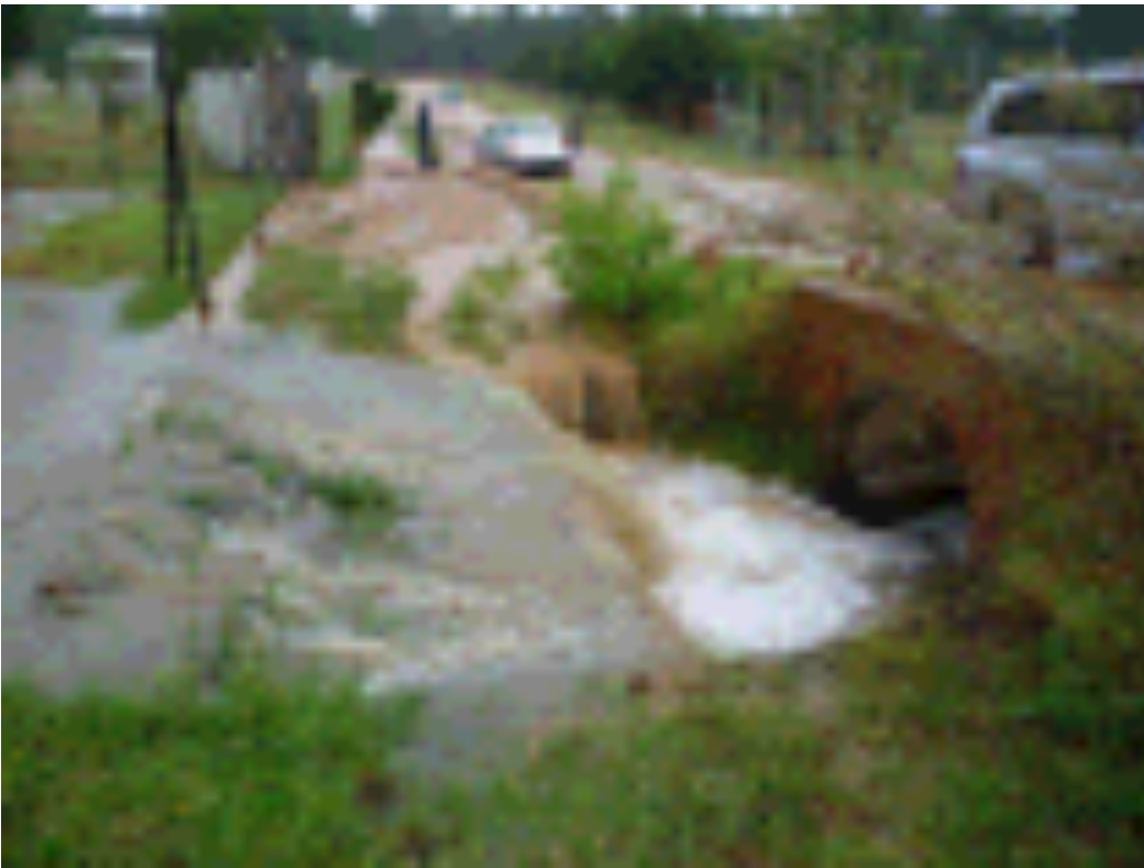
Figure 35 Sedimentation (on road verge) and storm water on Macintyre road following on a storm event on the 31 st of January 2014
