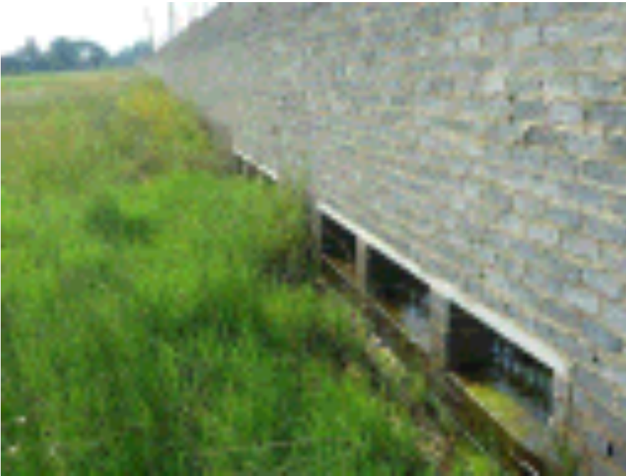
Figure 25 Northern boundary of the site with water running off from the upslope site to the north.
