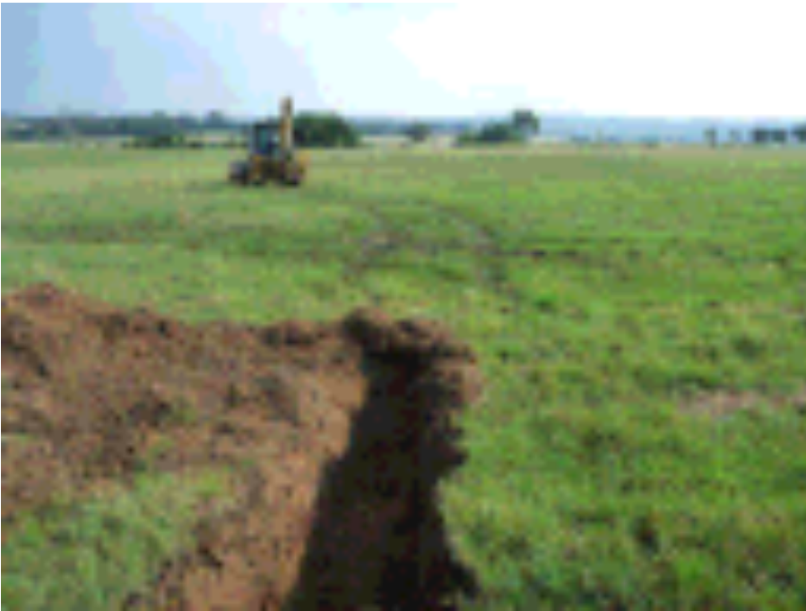
Figure 26 Profile pit on the northern boundary of the site (filled-in area) with signs of ponding water.
