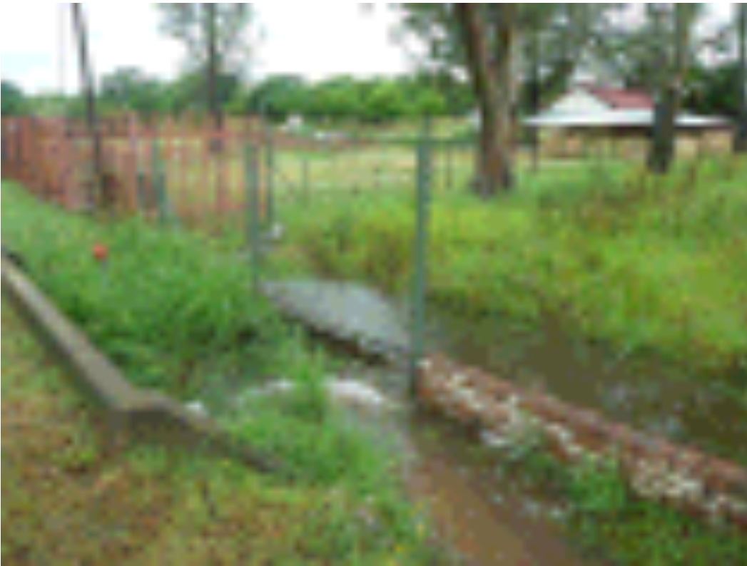
Figure 23 Culvert under Mc Innes road receiving water from the drainage line and surrounding properties (1 hour after a storm event on the 31 st of January 2014)
