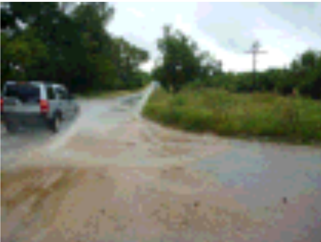
Figure 30 Storm water still present in Zinnia Road one hour after a storm event on the 31 st of January 2014
