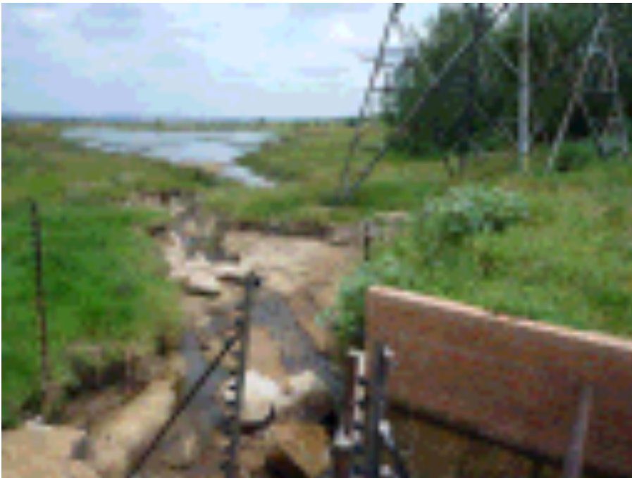
Figure 29 Eroded channel with distinct impacts on an Eskom pylon.
