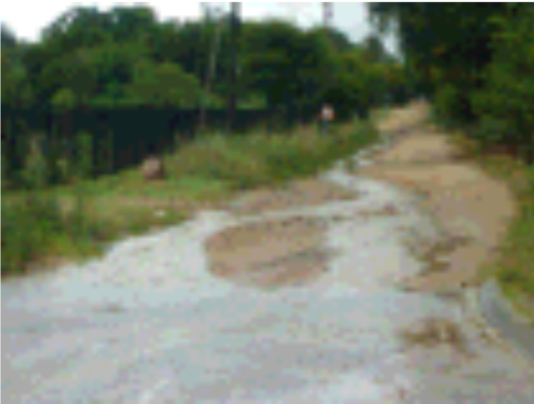
Figure 31 Storm water running down Rena Road one hour after a storm event on the 31 st of January 2014
