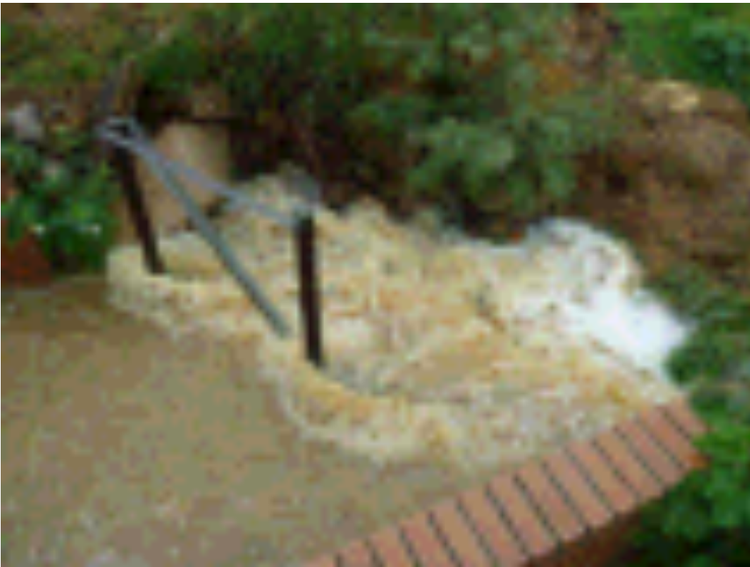
Figure 35 Storm water outflow
