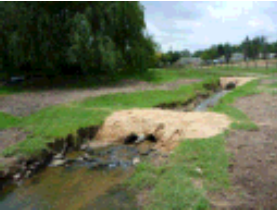
Figure 30 Eroded channel with newly constructed structures to prevent further erosion.
