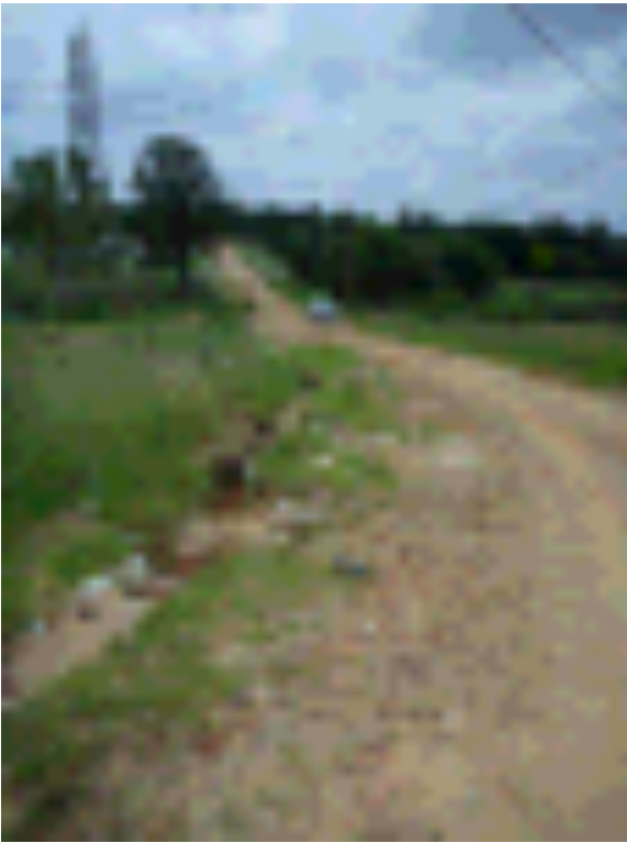
Figure 46 Erosion on the dirt road boundary of the site. This is the main source of the sediment in the impoundments.
