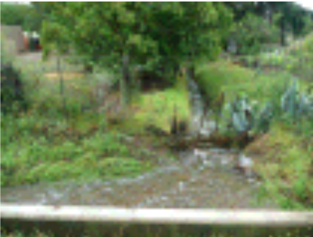
Figure 24 Culvert under Mc Innes road releasing water into the trench on Holding 32 (1 hour after a storm event on the 31 st of January 2014)
