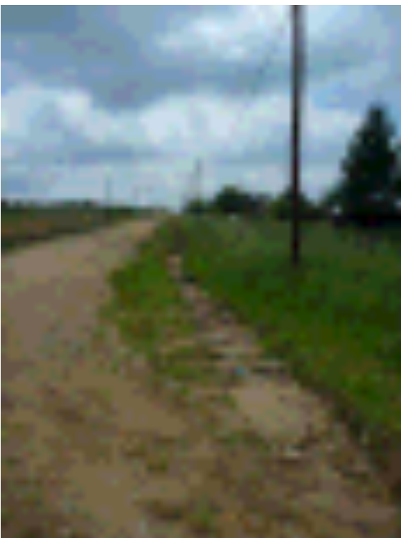
Figure 47 Erosion on the dirt road boundary of the site. This is the main source of the sediment in the impoundments.
