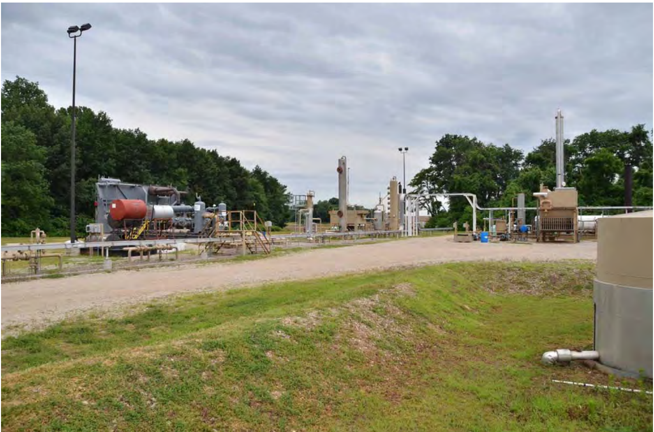
Plate 3.13: An example of a typical gas processing facility (Photo: Richard Montjoie).
