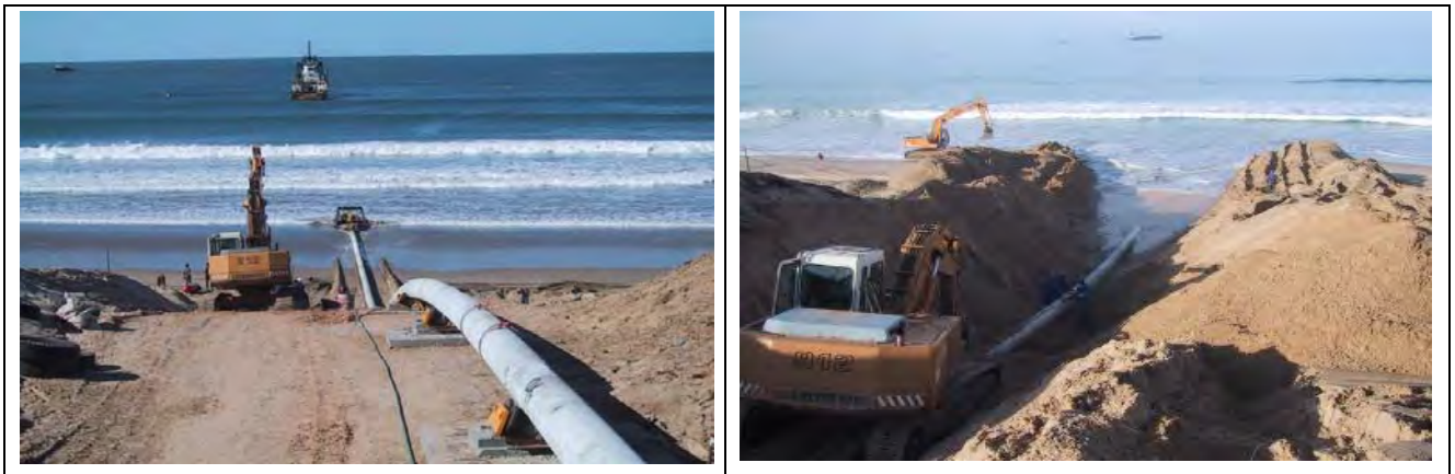
Plate 3.15: Examples of a trenching and bottom tow installation method (Source: Murray & Roberts Marine – Mossel Bay).
