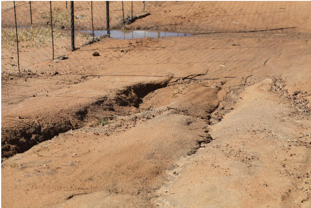
Photo 14 Erosion in the road and seasonal streambed crossing the road at Streamcrossing No3 at the site. Photo: R.F. Terblanche
