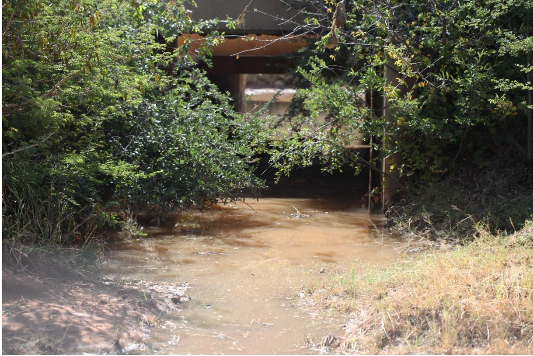
Photo 13 Culvert of Streamcrossing No3 at the site. Water visible in picture gathered after substantial rains. Photo: R.F. Terblanche
