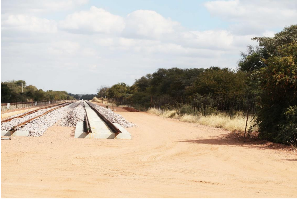
Photo 1 View existing railway and railway reserve at part of the site. Photo: R.F. Terblanche
