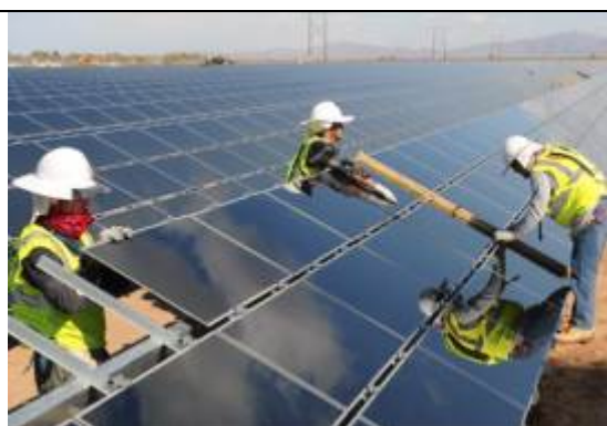
Figure 2.4: Picture of the installation of a typical PV array (courtesy of First Solar, Inc)
