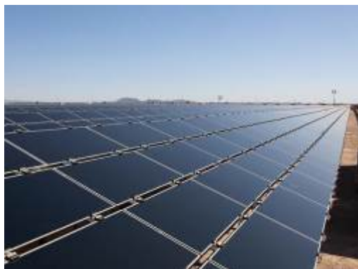
Figure 2.5: Picture of a typical PV array
