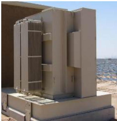
Figure 2.7: Photograph of a typical transformer (courtesy of First Solar)
