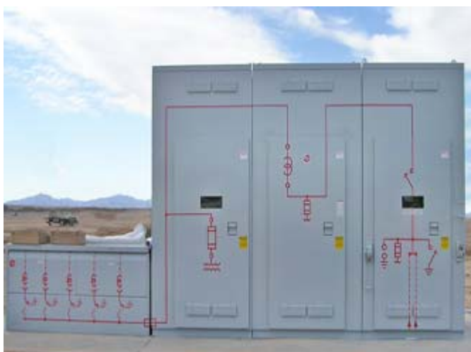
Figure 2.8: Typical PV Combining Switchgear Cabinet
