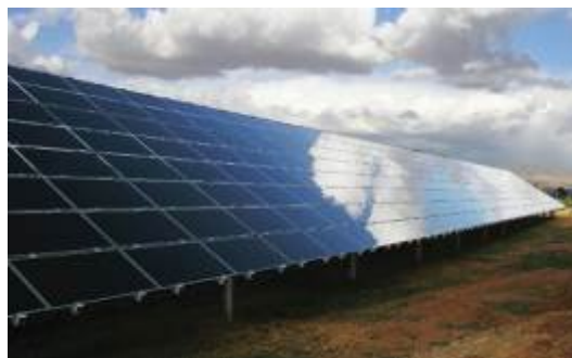
Figure 2.6: Picture of a typical PV array
